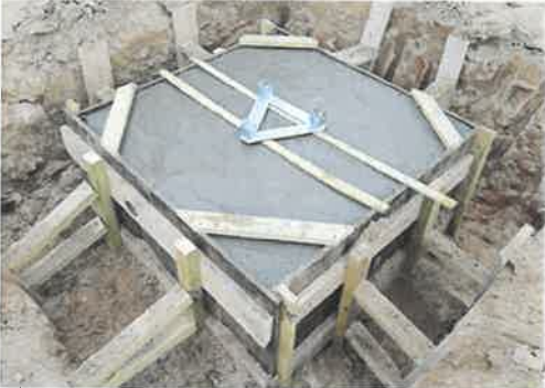
The fresh concrete foundation of the tower with the embedded anchor bolts and the base mounted on them
