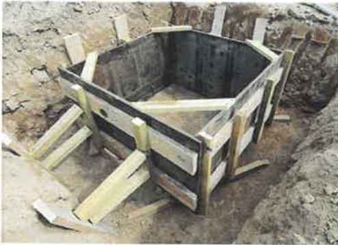
View of the form work for the foundation of the MK tower
